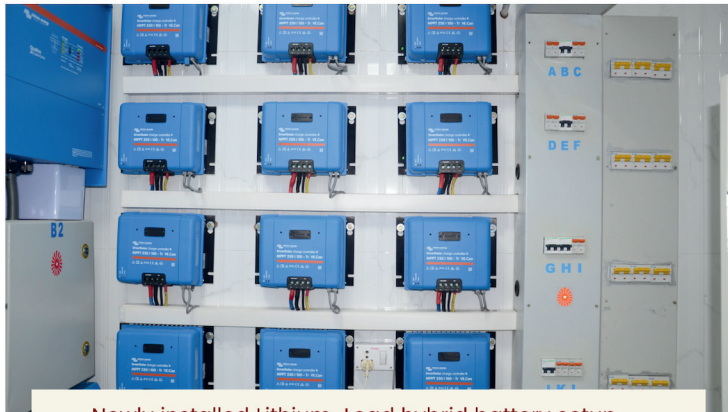
Newly installed Lithium-Lead hybrid battery setup
